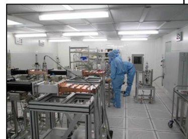
EU-XFEL : Preparation and power testing of 800 couplers
