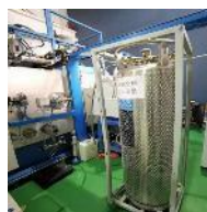
N2 Cooling system
