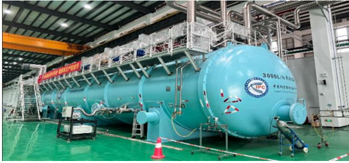
Figure 5. CEPC 18kW@4K cryogenic refrigerator.
