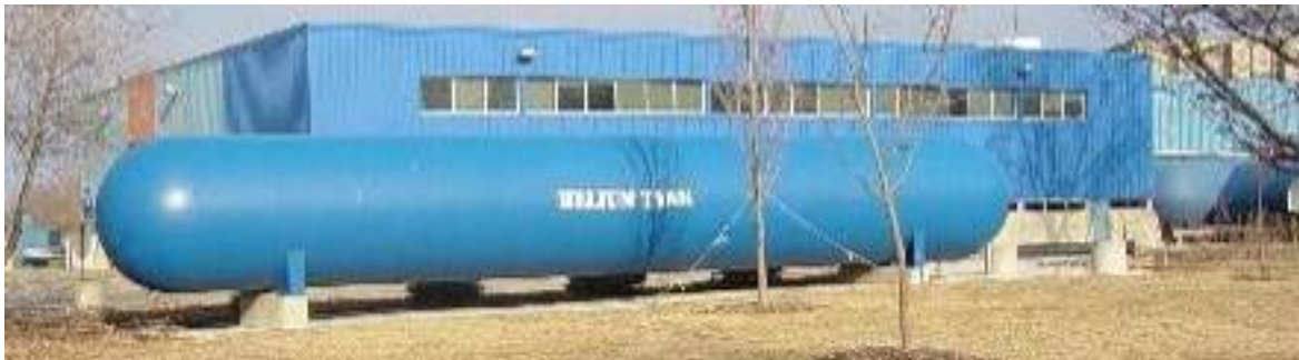
Figure 16: Example of a 30,000 gallon GHe storage tank
