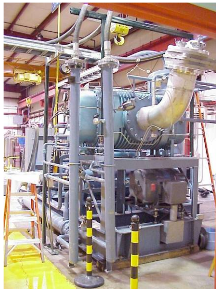
Figure 15: ILCTA_MDB Kinney Pump
