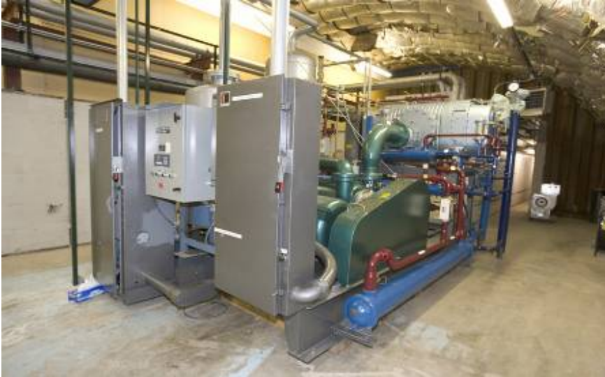
Figure 4.2 Large Vacuum pumps at MDB
