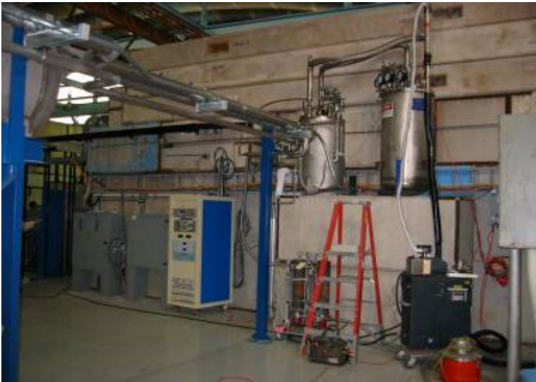
Figure 4.3 Part of the new Cryogenics infrastructure at MDB
