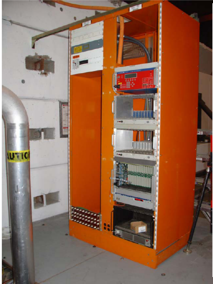
Figure 2: New ILC-ESA DAQ racks in ESA are installed on the outside of the beamline concrete bunker. Rack B061-02 contains a slave VME crate, connected by fiber optics to the master VME crate in ChA; a Camac crate; 2 NIM crates and a C.A.E.N. HV crate (48
