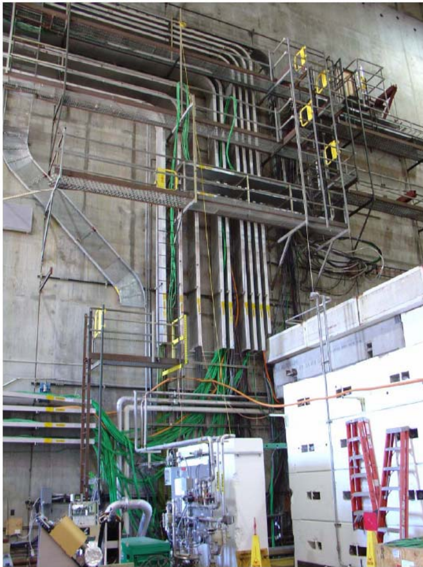
Figure 8: Cable Trays on West Wall of ESA
