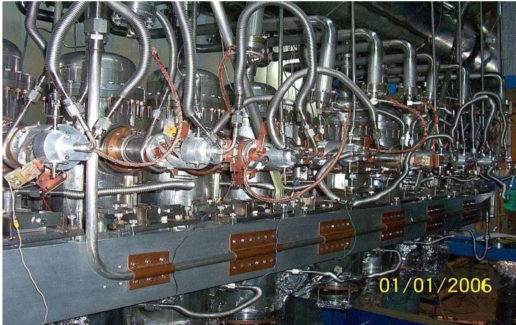
8 QWRs and superconducting solenoid in Linac module 1
