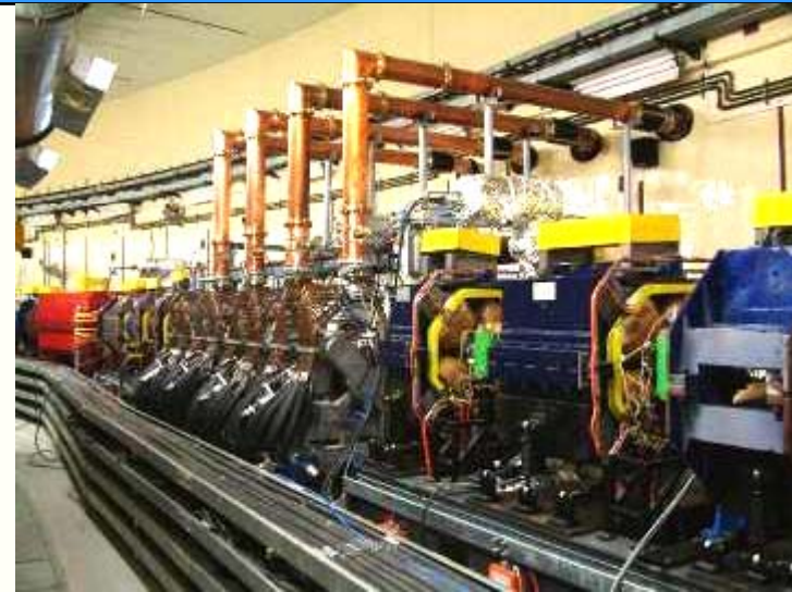
RF Cavities installed in Indus-2 Ring
