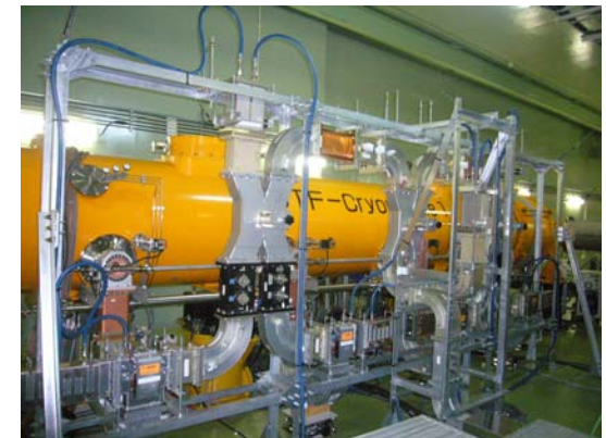
high power test, with 4 cavities
