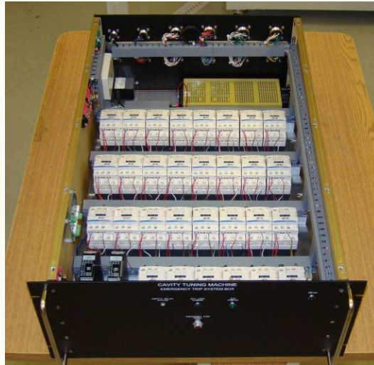
Emergency Trip System Box
