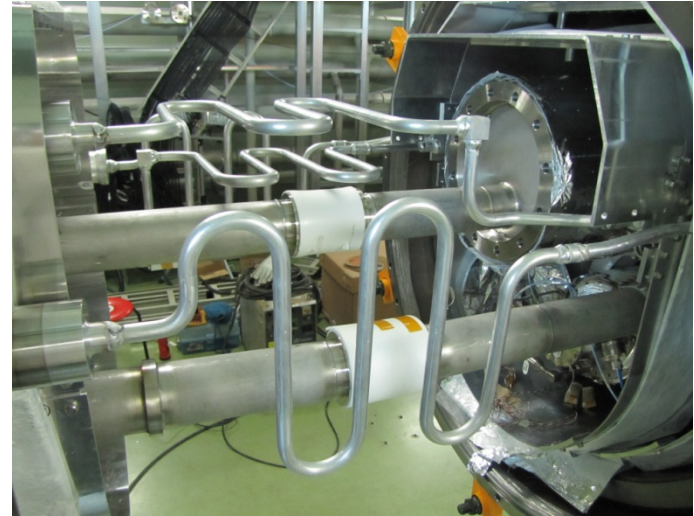
Cooling pipes between Module-C and Module-A
