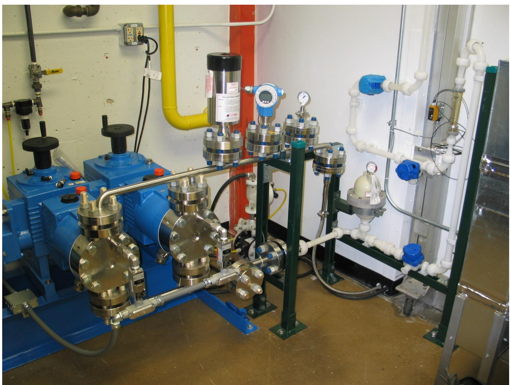
HPR system in IB4
