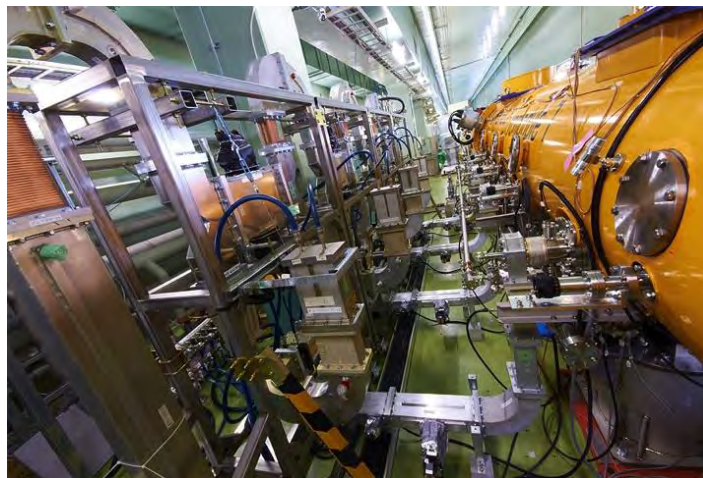
Figure 4-10: Experimental apparatus used for RF conditioning with a high-power RF source in Cryomodule-A.
