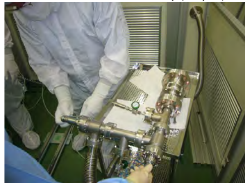
Figure 7-5b: Transition piece leak check.
