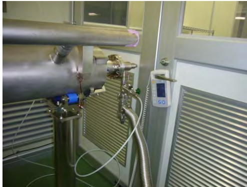
Figure 7-6a: Cavity Z109 assembled with the new flange/valve assembly at the beam pipe flange at the non coupler end of the string.
