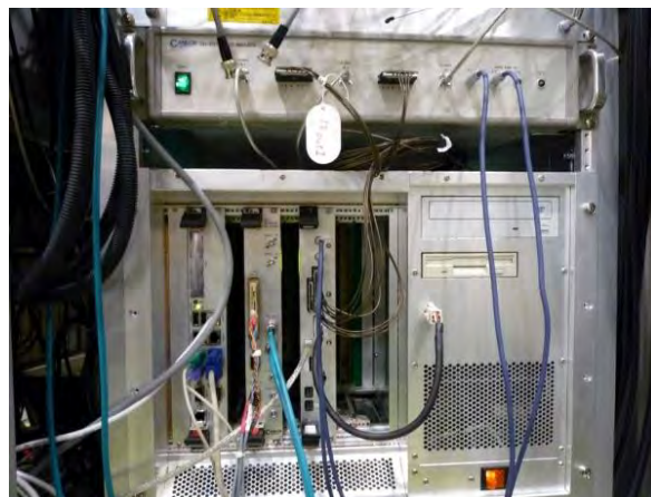
Figure 10-2: Photograph of the cPCI digital FB system.
