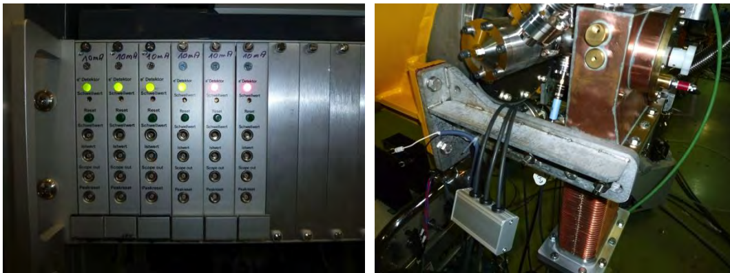
Figure 4-5: Electron interlock system for coupler protection supplied by DESY.
