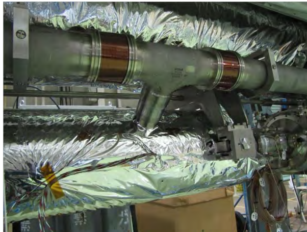
Figure 7-28: The cross connect pipe between the KEK cavity jacket and LHe supply pipe. A Ti-SUS junction pipe was used as the cross connect pipe. The two stainless steel bellow pipes were connected to this pipe.
