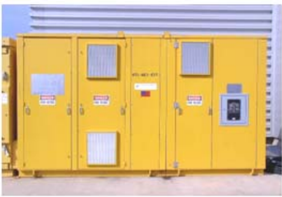
RECTIFIER TRANSFORMER AND FILTERS
