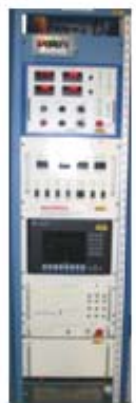
EQUIPMENT CONTROL RACK
