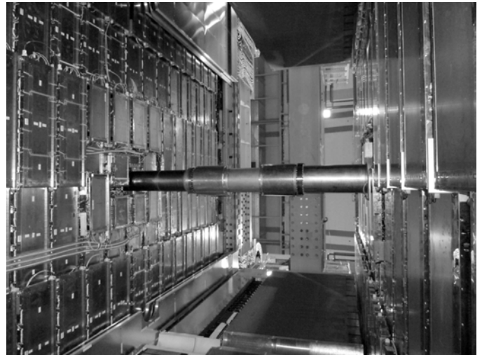
Fig. 3. View of the M1 (left) and M2 (right) LHCb Muon Stations from the cavern floor, with the Calorimetric System is in the open position.
