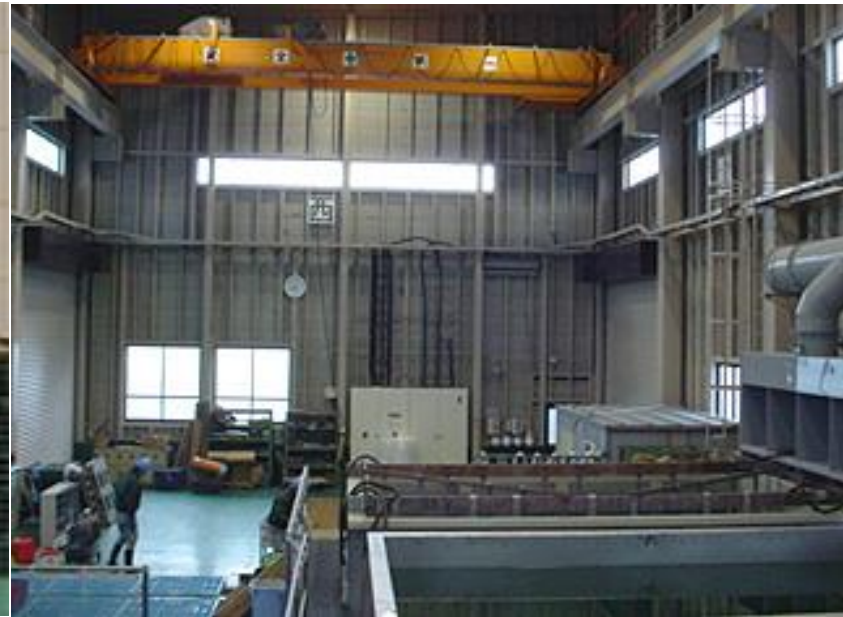
The electrolytic polishing plant inside
