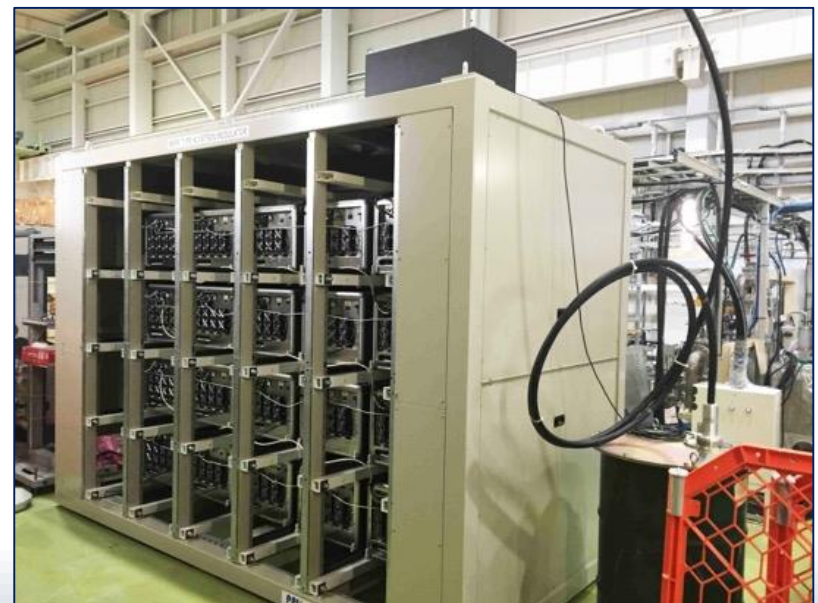
20 KEK-Marx Unit combination for 120kV.
