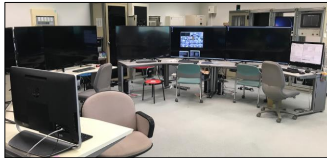
STF control room
