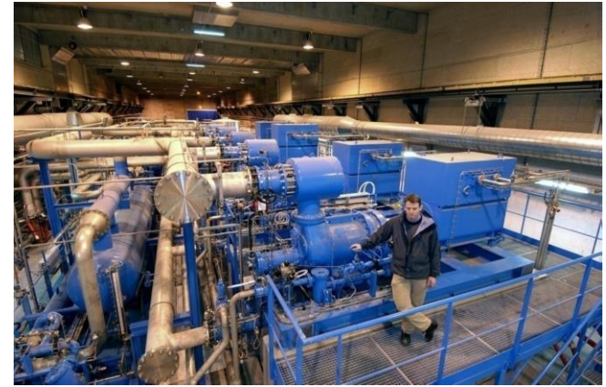
CERN cryogenic plant
