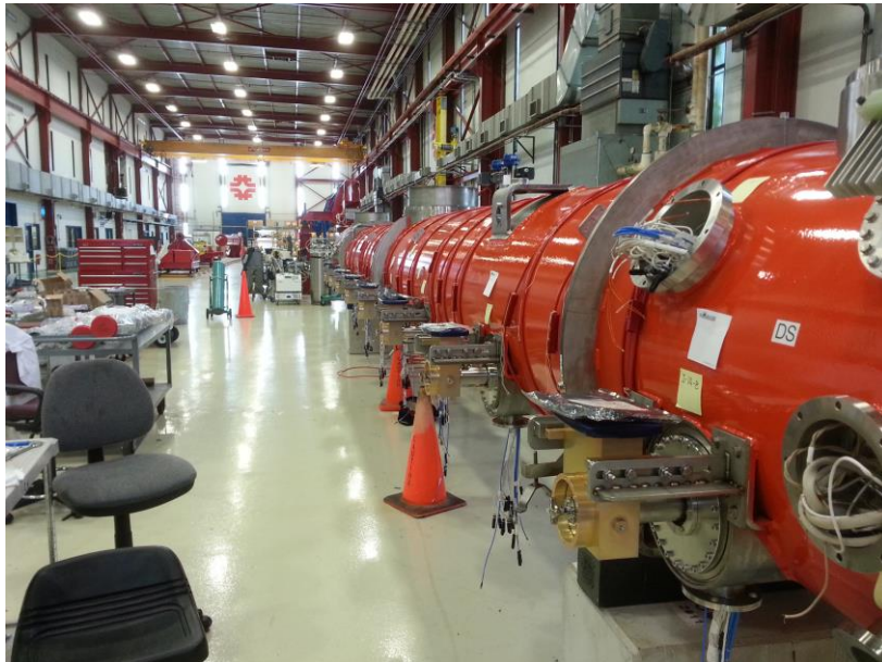
pCM with all eight FPC's installed
