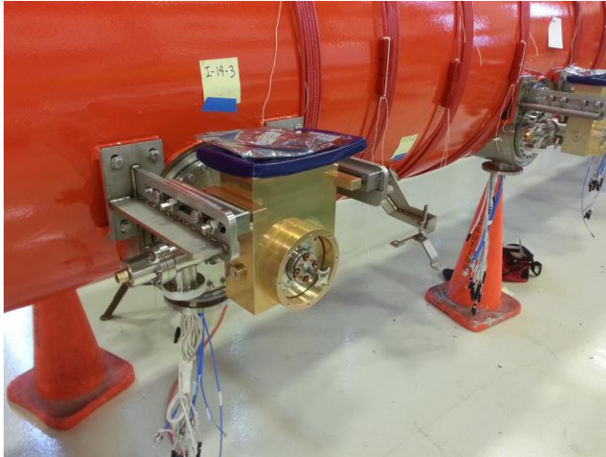
FPC installed with waveguide box (manual adjustment knob)
