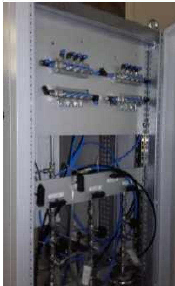
RPC gas recycling system
