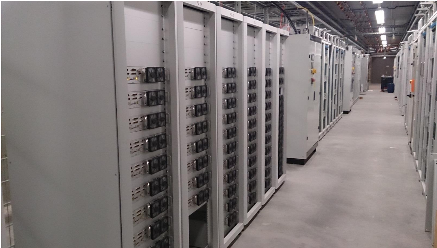
power supply room XFEL injector
