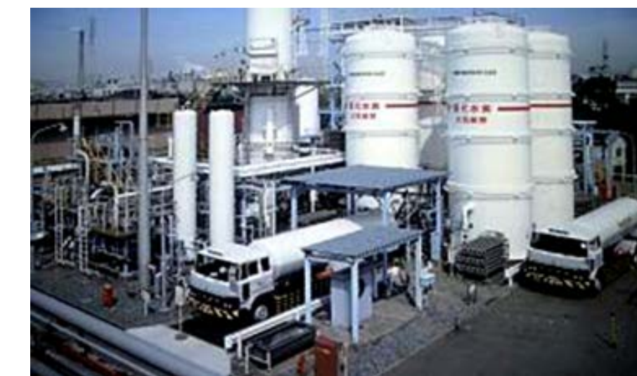
Photo 4: Vertical cylindrical tanks
